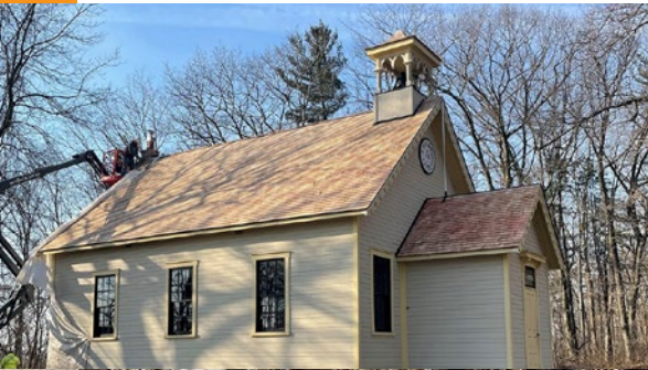
The cedar shingle roof of the historic Rokeby School at Lambton Heritage Museum is replaced as part of ongoing restoration work.
