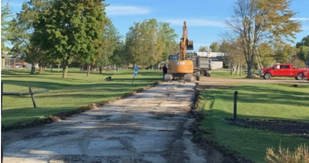
Workers prepare a new asphalt laneway as part of parking and site improvements at Oil Museum of Canada in September.
