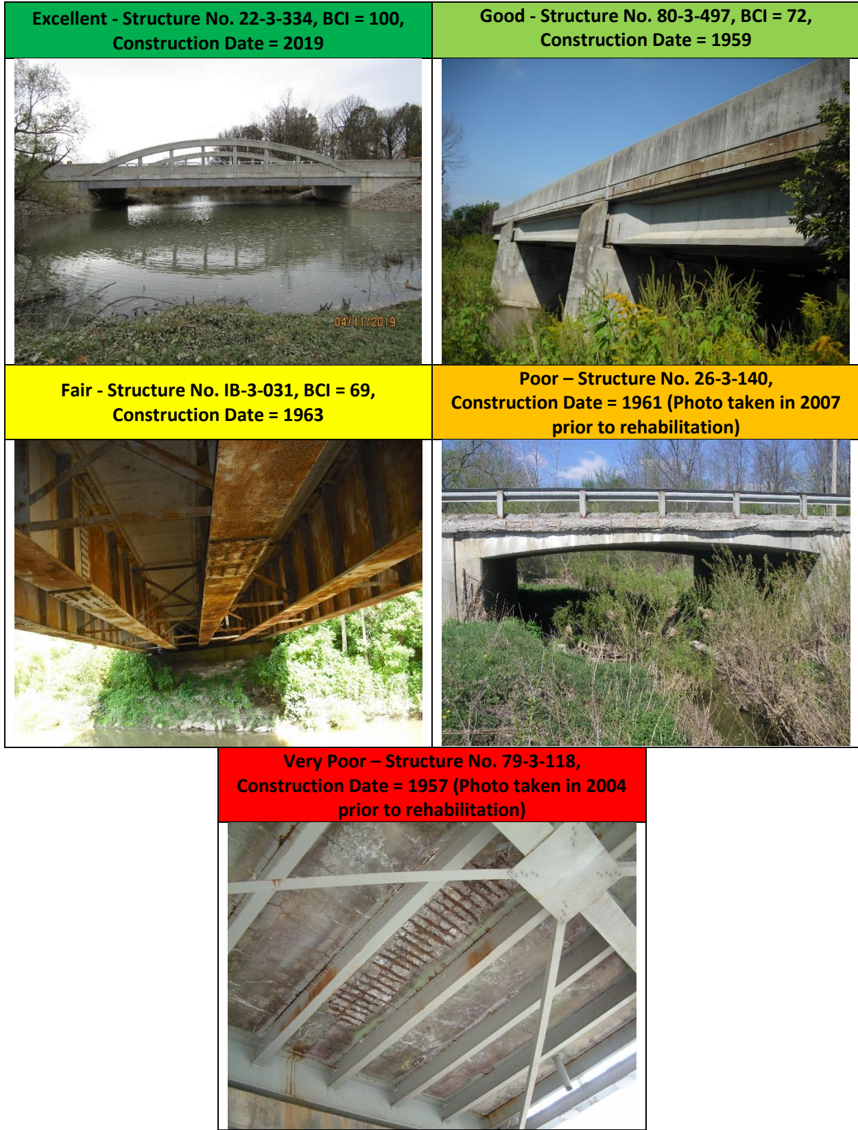
Figure 3-4: Local Examples of Bridge Condition
